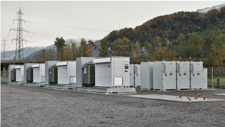
By Kecko from Eastern Switzerland - Walenstadt - Large Battery Storage, CC BY 2.0, https://commons.wikimedia.org/w/index.php?curid=140651440
